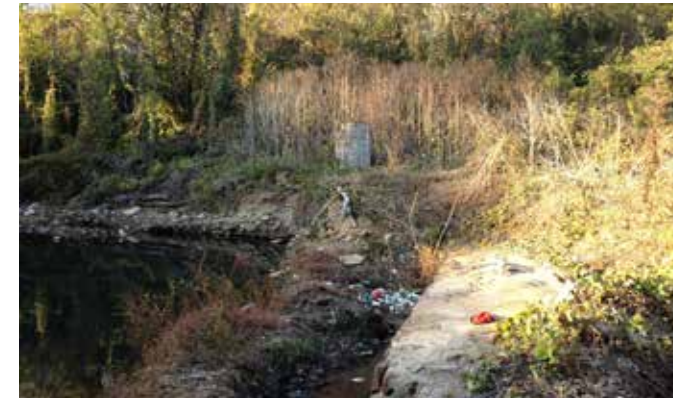
(1) Debris in Proctor Creek
