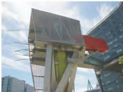
Portland, Oregon - Air Terminal
